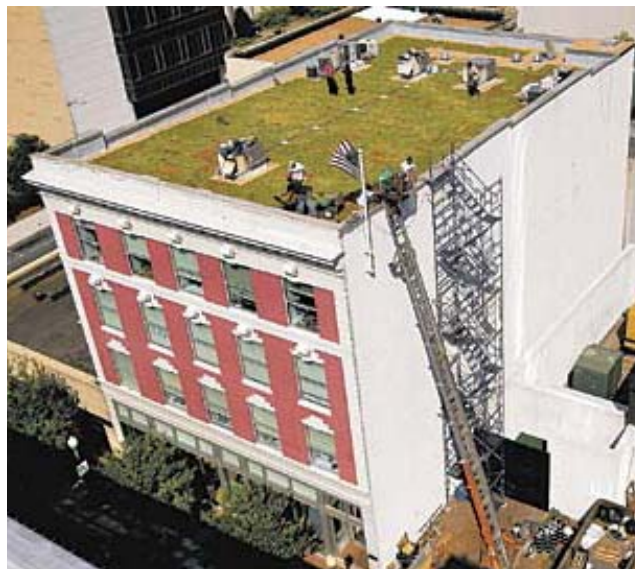
Above: April 2004 photo of the completed Atlantic Building green roof by Mort Fryman/The Virginian-Pilot.
