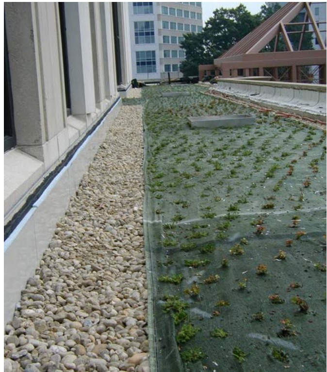
The newly planted green roof is on a former tar-and-gravel roof. Photo taken just after planting was completed in October 2003.
