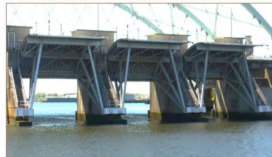
Example of existing Tainter gates at Fox Point Hurricane Barrier in Providence, Rhode Island
