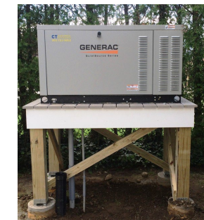
Elevated critical equipment
