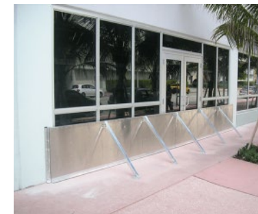
Temporary flood panels
